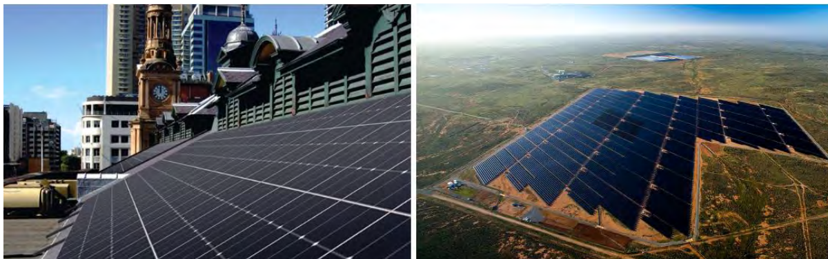
Solar panels on the Sydney Town Hall, and the 53 MW Broken Hill Solar Farm, which covers 140 hectares. Credit: Broken Hill, Jeremy Buckingham, Wikimedia Commons
